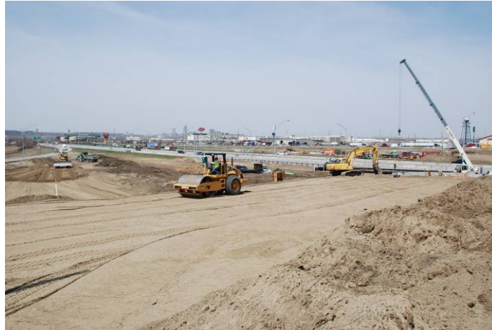
Figure 5. The location of the new bridge during stage 1 (Photo to the west of existing bridge)
